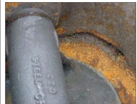
Fig. 31: Plant shutdown due to “quick and dirty” sizing with 8 inch rotary plug valve and too small DN.
