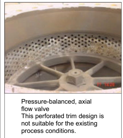
Fig 41: Insufficient commissioning and poor cleaning and flushing of the pipeline.
